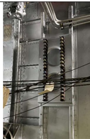
The Connection Panel, bomb-bay portside midship, has been re-manufactured and installed and is awaiting cables to be run and connected.
